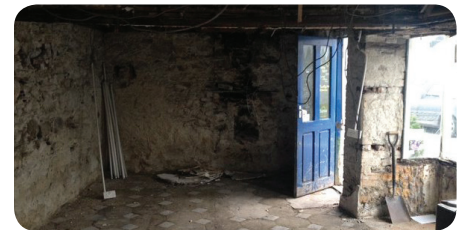
The gutted shop interior.
